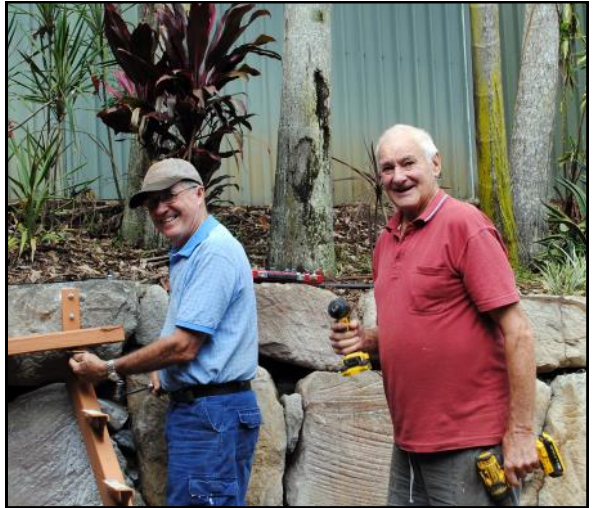
Rob Howard and Mal Longton building new steps up to the expanded Festival Shed.
